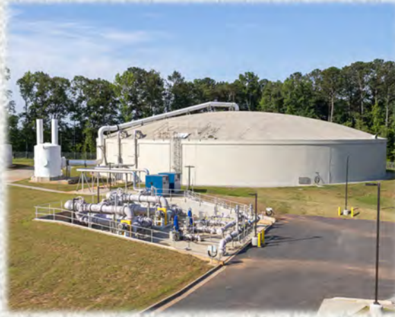
Water Treatment Facility
